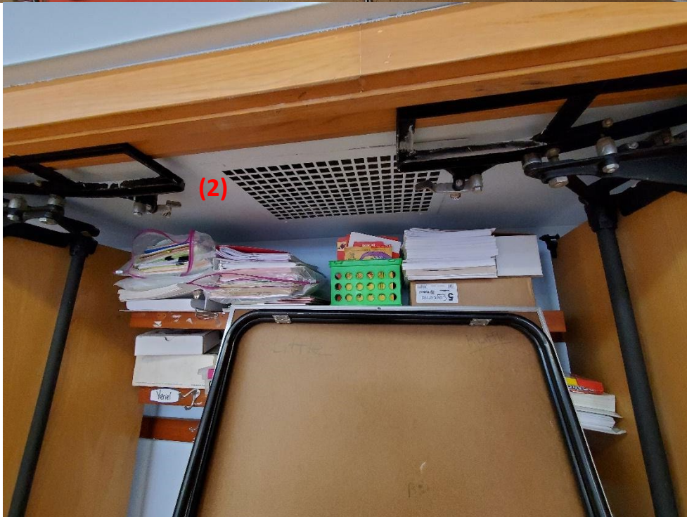
Typical mechanical ventilation setup in classrooms with (1) supply air vents on the soffit above the student closets and (2) a return located inside the student closet.
