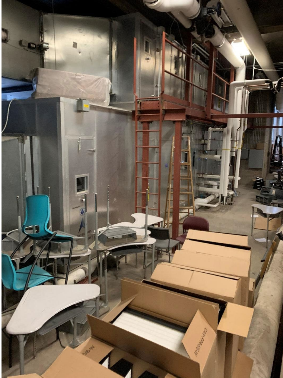
Air handler unit in Franklin Campus
