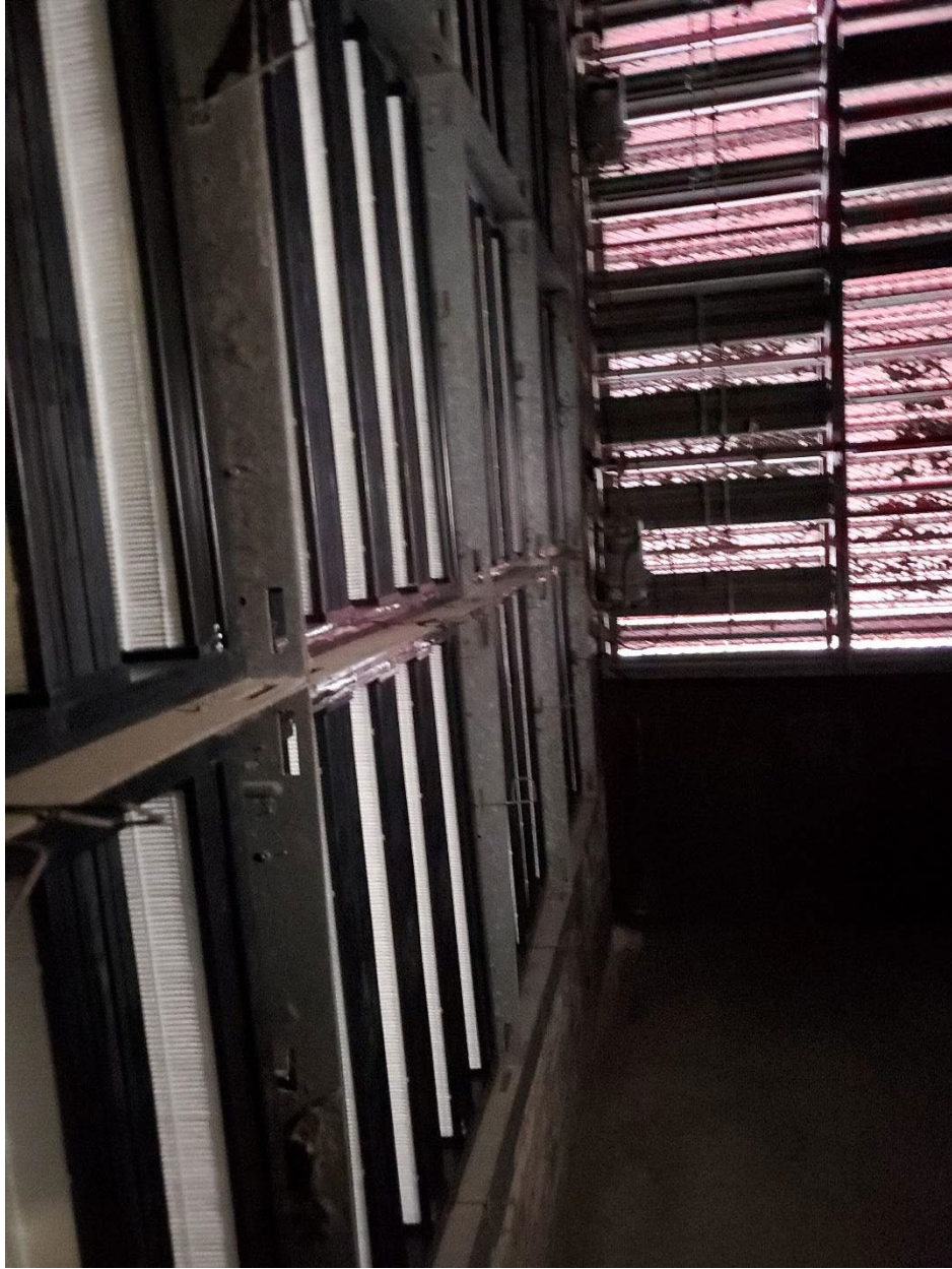
MERV-14 filters in filter bank. The outside air dampers are opened.
