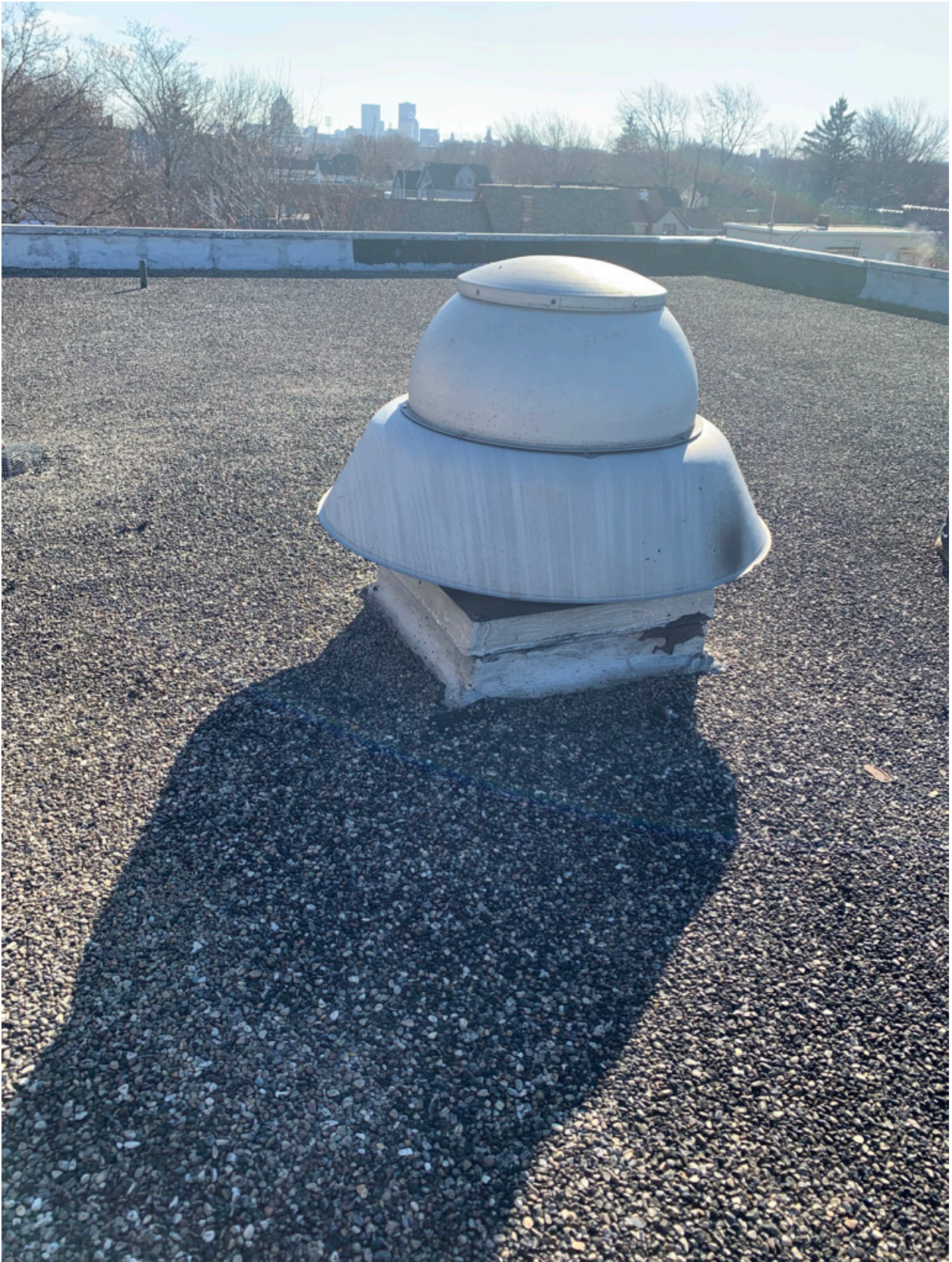
The roof top exhaust fans should be inspected and repaired where not working
