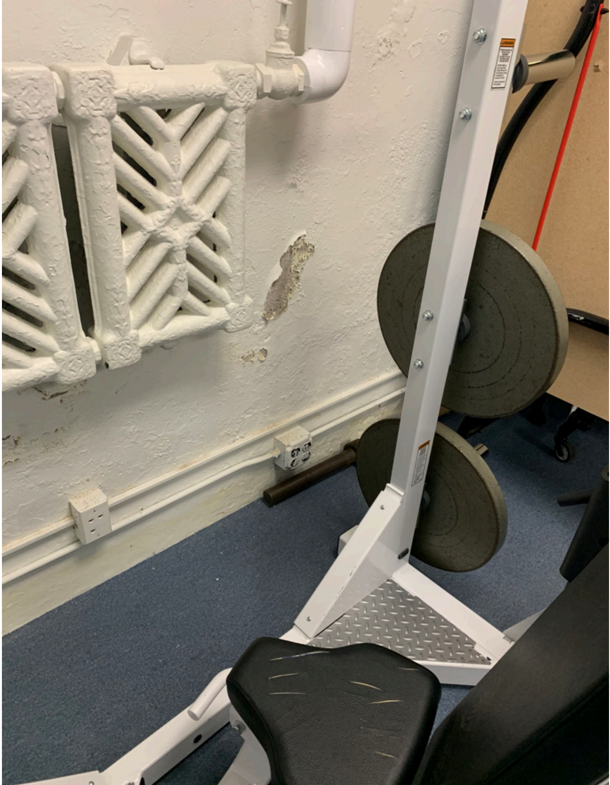
there is dampness in the foundation wall in the weight room and this has caused a musty odor in the carpet.
