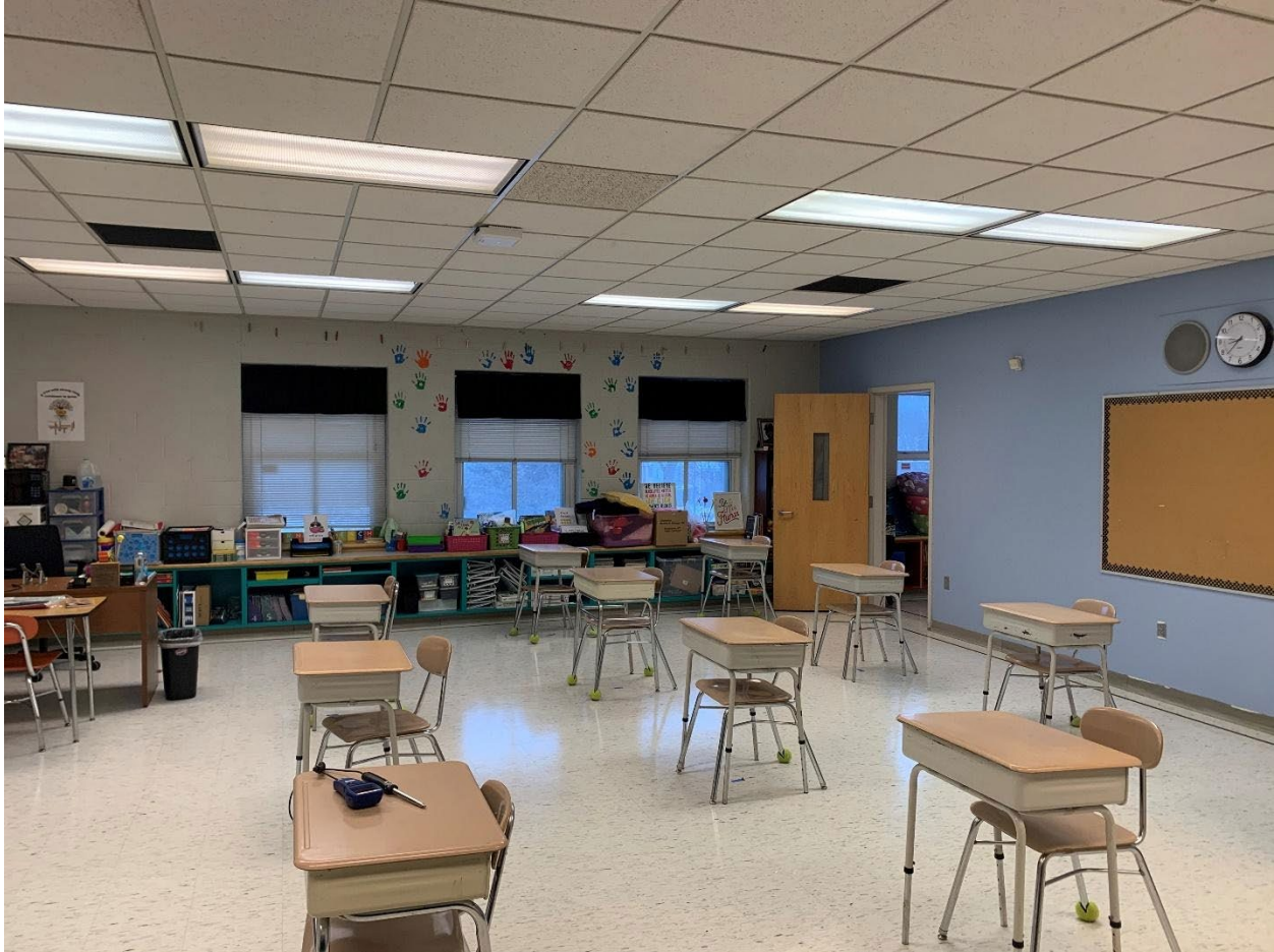
Standard ventilation scheme in classrooms. Operable windows for natural ventilation with mechanical ventilation supply located around the light fixtures and passive return into the ceiling.
