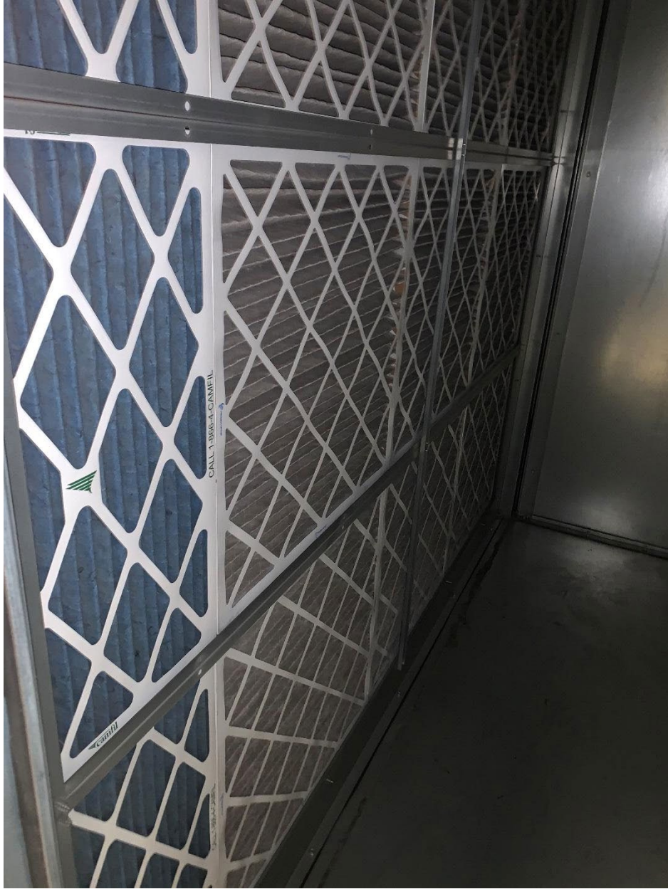
Mixing box inside air handler units. MERV 8 filters installed.
