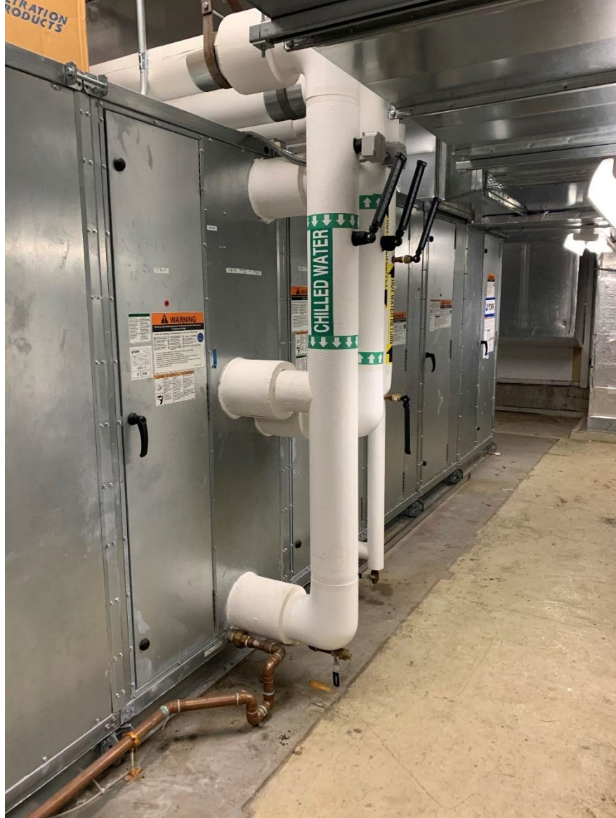
Standard air handler unit serving the building.
