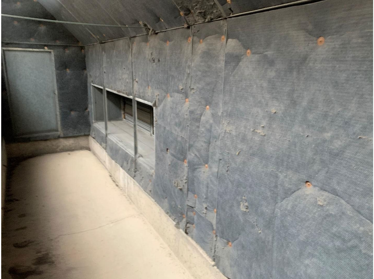
Outside air plenum in an air handler unit. The outside air dampers is minimally open due to temperature constraints.
