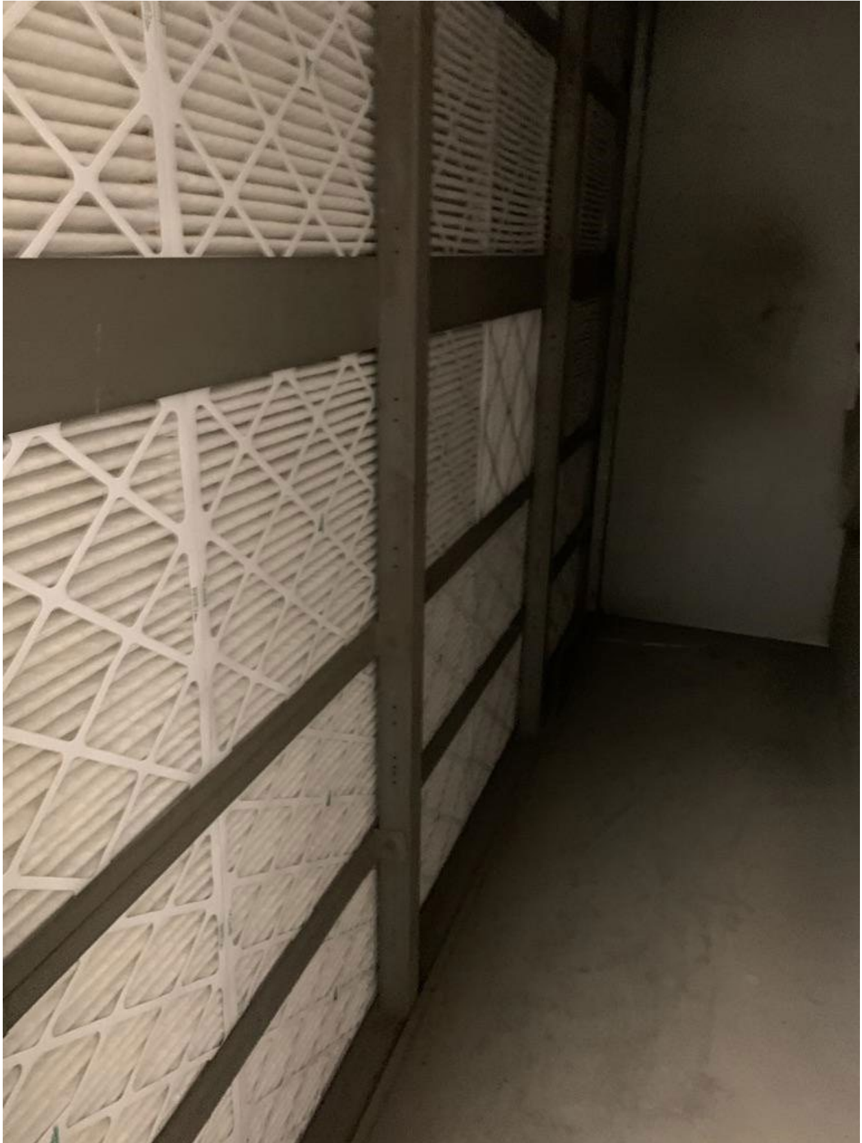
MERV 13 Filtration in air handlers
